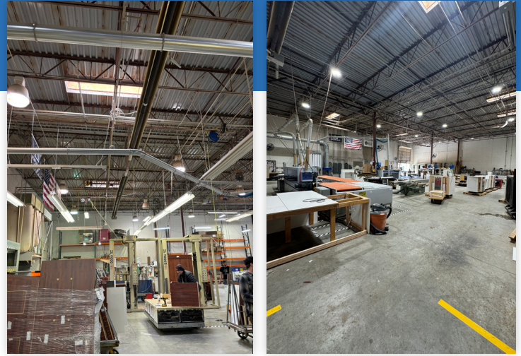
Lighting Project Before & After
